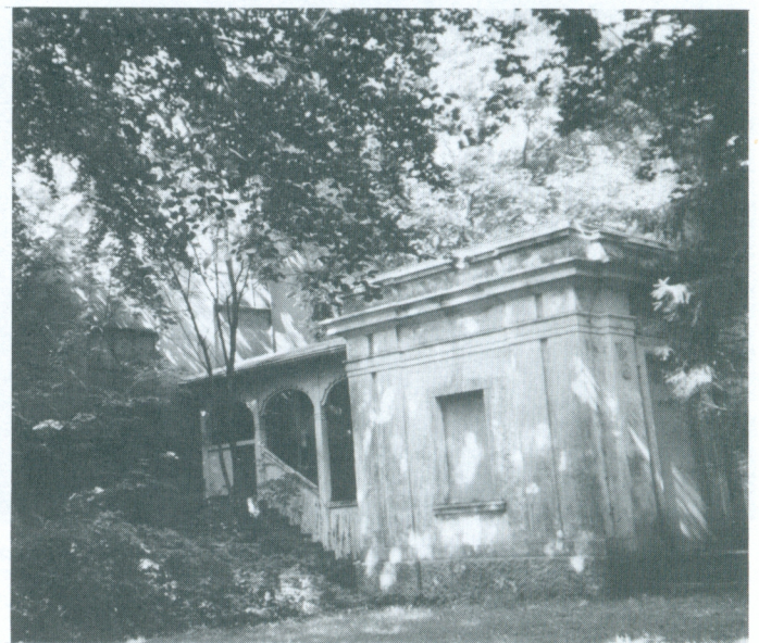
The classical style entry and rustic stairway to the telescope's housing reveals 19th century interest in "gesamtkunstwerk" (a complete artwork), even for an Observatory.
